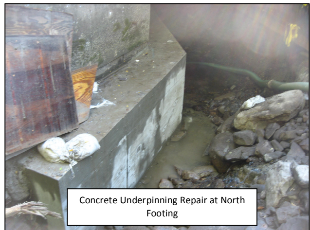
Undermining and Scour at North Footing
