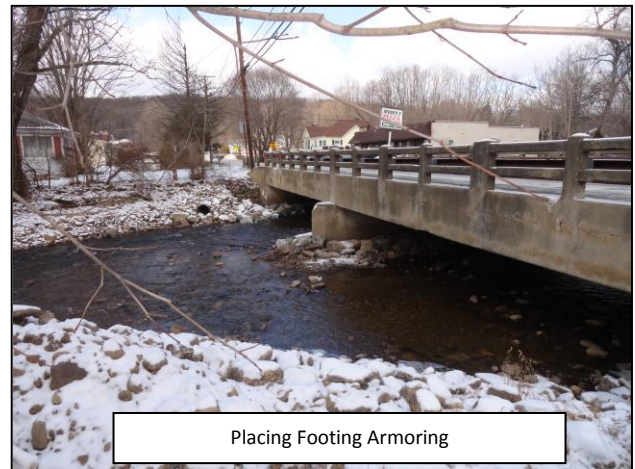
Debris Build Up Under Bridge Prior to Cleaning
