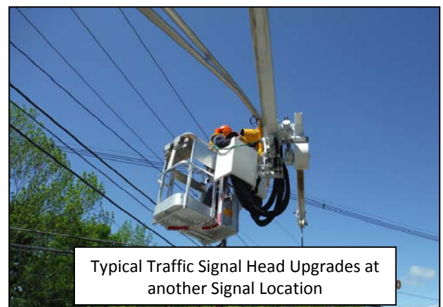
CR-622, Looking East towards Signal SC-06 and CR-519
